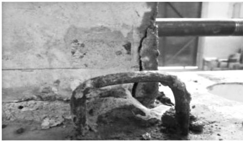
图6 试件WS-4至WS-15破坏现象典型实例 Fig.6 Failure phenomena of the specimens ws-4 to ws-15
